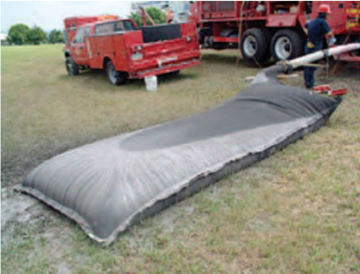
Figure 6-2. Typical Example of Settlement Tanks
